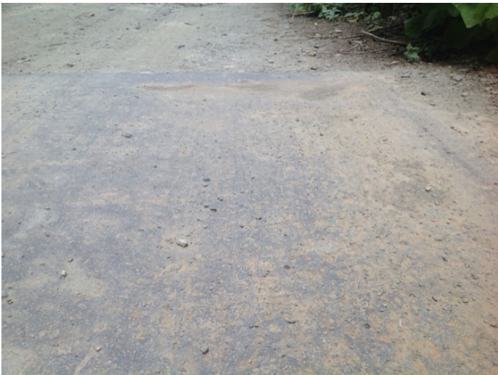
steel plate damage
